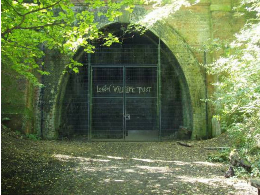
Entrance to the railway tunnel in Sydenham Hill Wood LNR (Now a bat registered roost).
